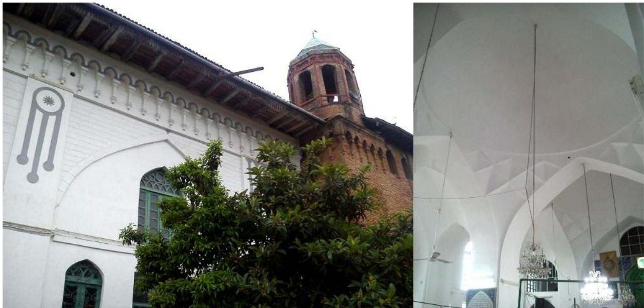
Figure 1- Difference between the internal and external form of the roof of Akbarieh Mosque in Lahijan (Source: Authors)
